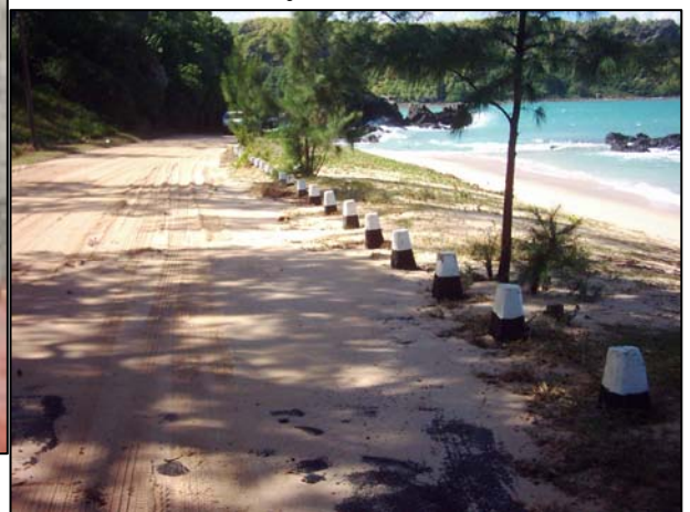
An estimated 3 – 5 tons of sand accumulation along the coastal road at Baie du Cap
